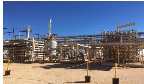
Figure 2: Membrane Installation at the Customer Site in West Texas
